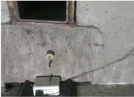
a) Propagation of crack
