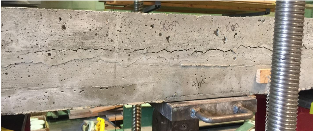
Figure 89. Case 4 positive bending flexural test specimen failure at concrete bond interface
