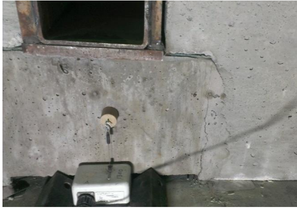
a) Propagation of crack
