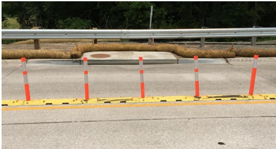
Figure 46. Manhole discovered near the approach to the westbound lane
