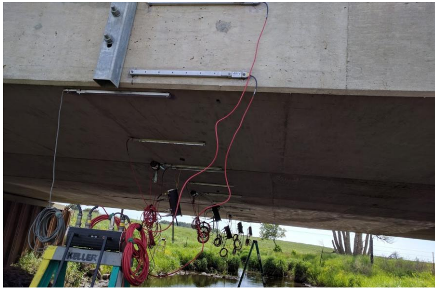
Figure 28. Instrumentation mounted on the bridge
